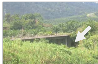
Arrow shows eroded cavity under Ombe Bridge
