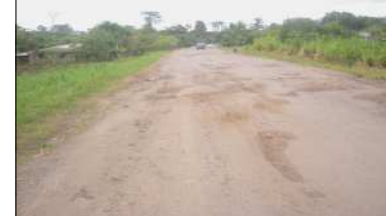
The dilapidated Mutengene-Kumba Road
